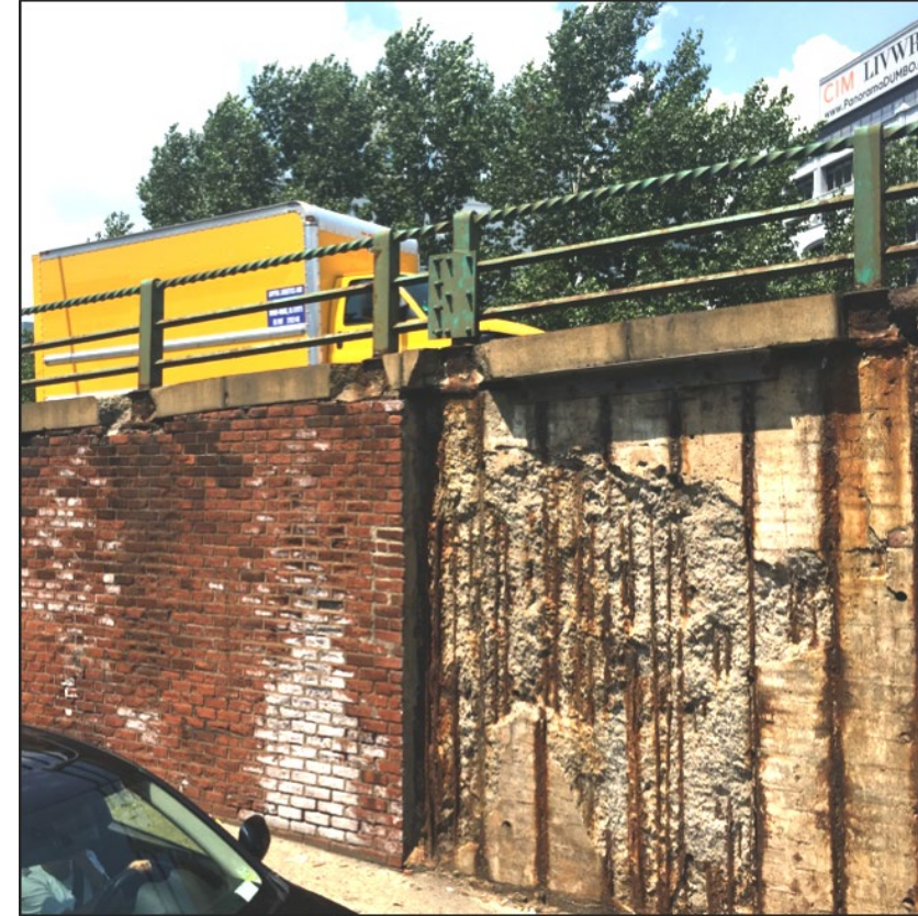
Exposed Reinforcing Bars Guard Rails Unsupported Walls Weakened
