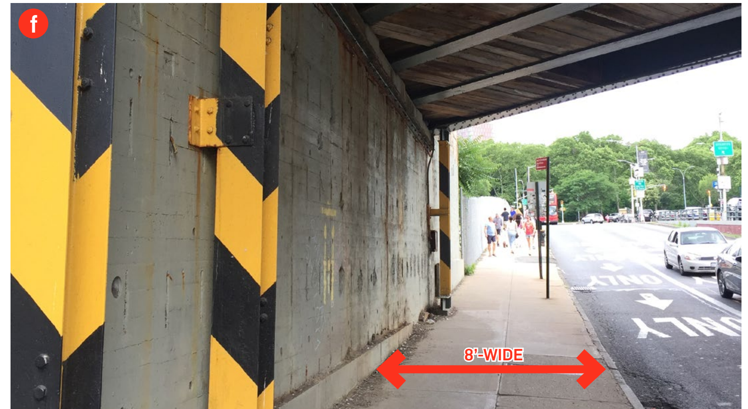
narrow and dark sidewalk under BQE
